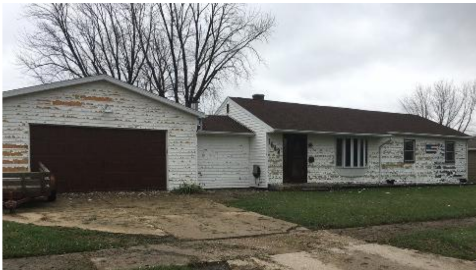
Hail damage seen on a house in Janesville, Wis. after a severe storm came through the area Wednesday night, May 2, 2018. (JennaMiddaugh/WISC-TV News 3)
