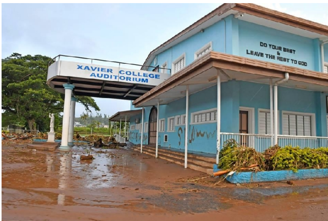
Damage caused by Tropical Cyclone Josie in Fiji, April 2018. Photo: Government of Fiji
